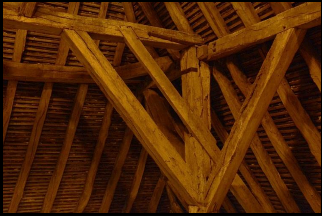
Figure 18: A detail of the structure in the Wheat Barn at Crossing Temple.
