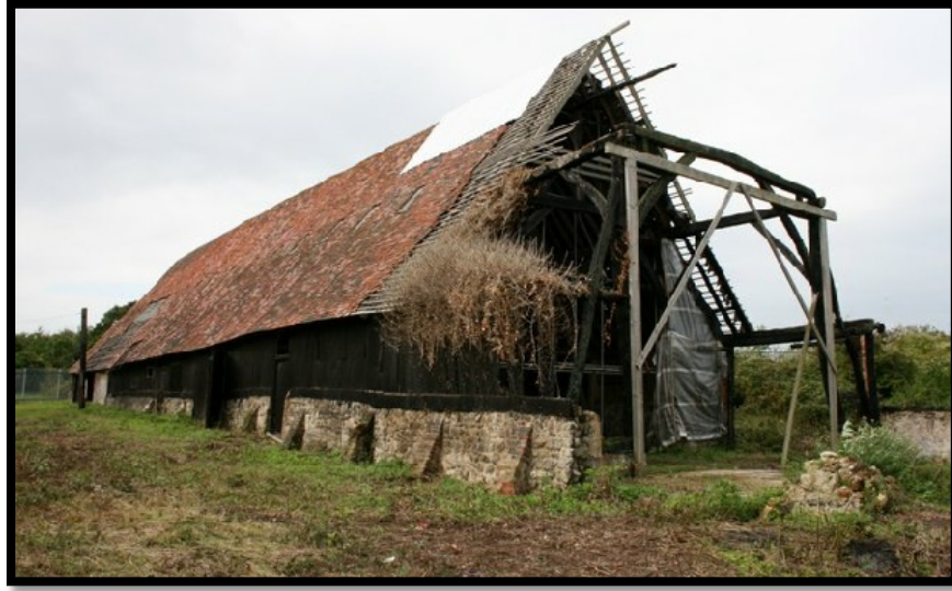
Figure 20: Frindsbury barn after it sustained fire damage in 2005.
